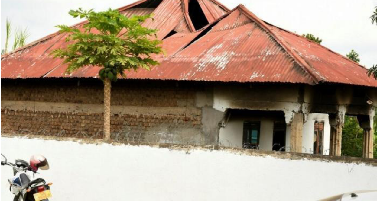
The burned-out shell of a dormitory at Lhubiriha (Mpondwe) Secondary School in western Uganda, photographed after the June 16, 2023, attack.
